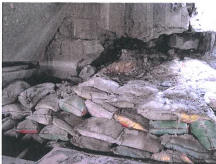
桥台锥坡坍塌
